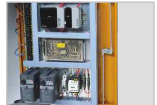
PLC (Programable logic controller) and High Quality Electrical Components
